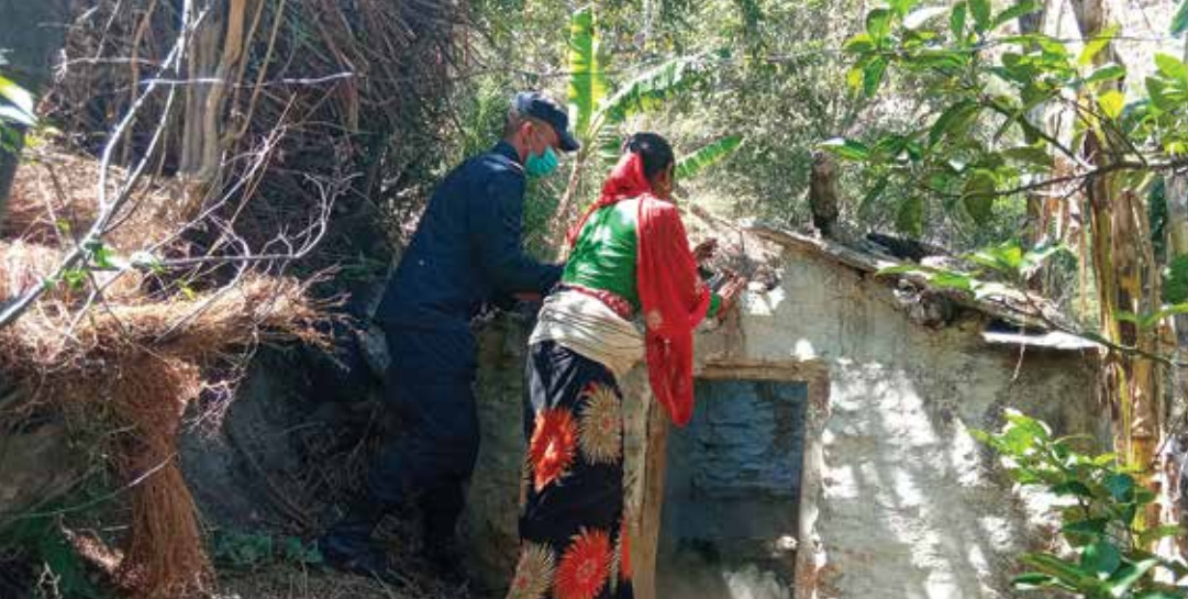
Receiving support from security personnel and Government stakeholders to demolish Chhaugoth, Bajura
