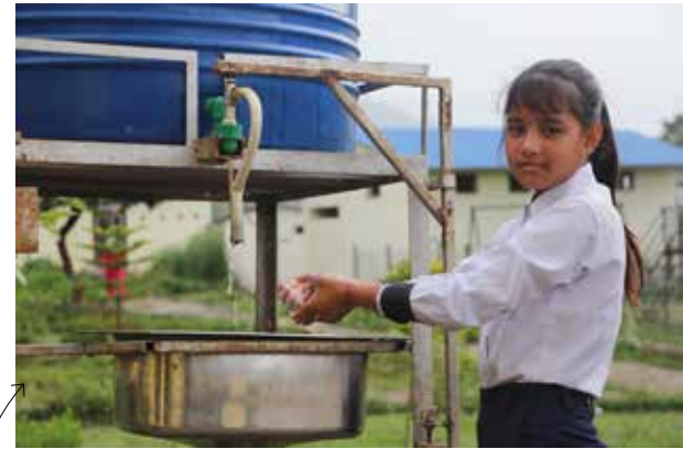
Clean hands, healthy kids! Thanks to the addition of a handwashing and drinking water station at school, children are now better equipped to maintain their hygiene.
